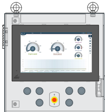
Figure 4-4-7: Local operating panel
